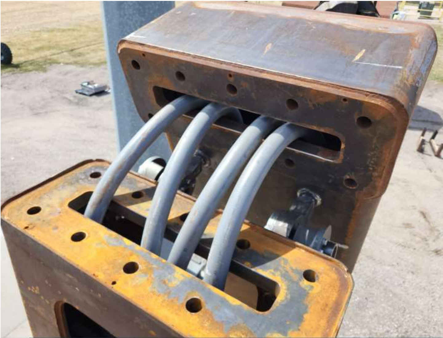
View of 2" Conduit
