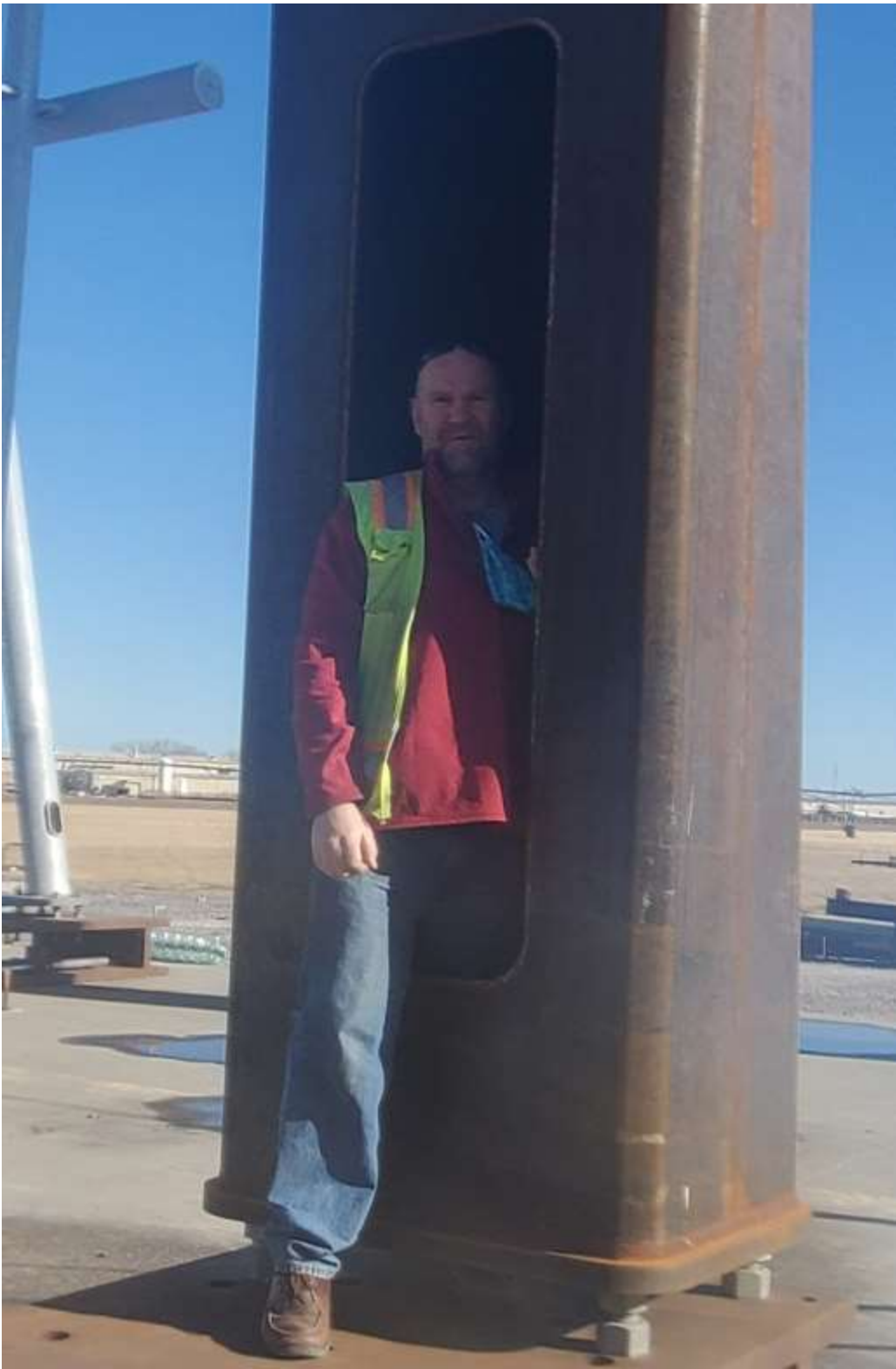
Equipment access opening at Pole Base (6'3" Person)
