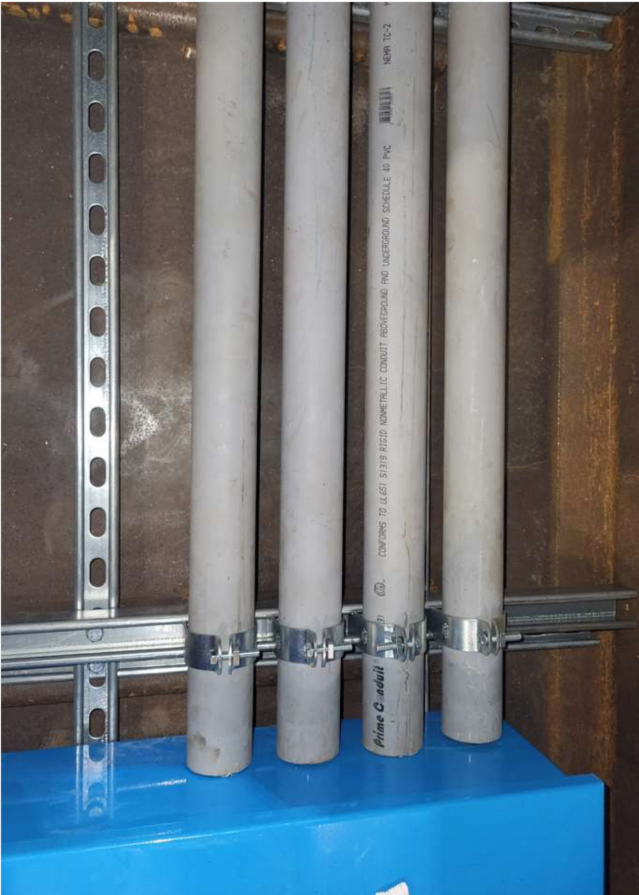
View of electrical cabinet
